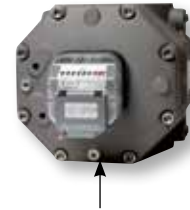
Oil level sight gauge
